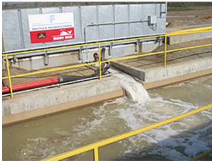
Figure 2: Water Recycling Tank
